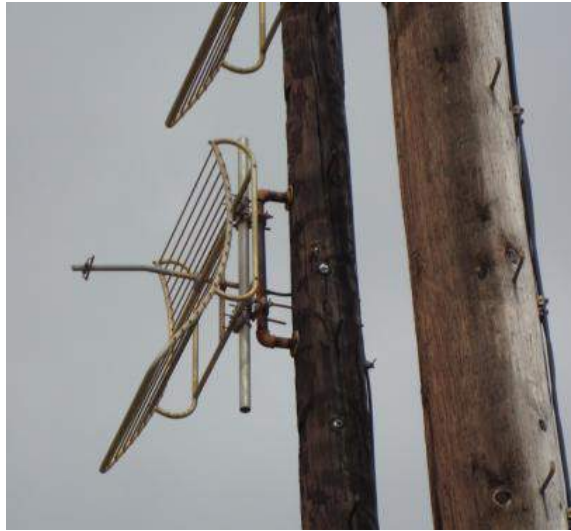
Two dishes remained attached to the poles but the ones that fell killed the satellite receive dish.
