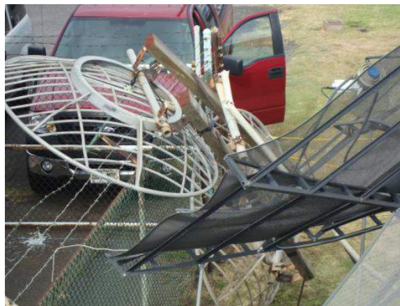
A nasty storm caused two STL dishes to fall down through the satellite receive dish
