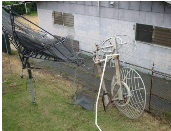
Viewed from another angle, not only is the damage visible, but we can see how close it was to where it might have hit someone.
