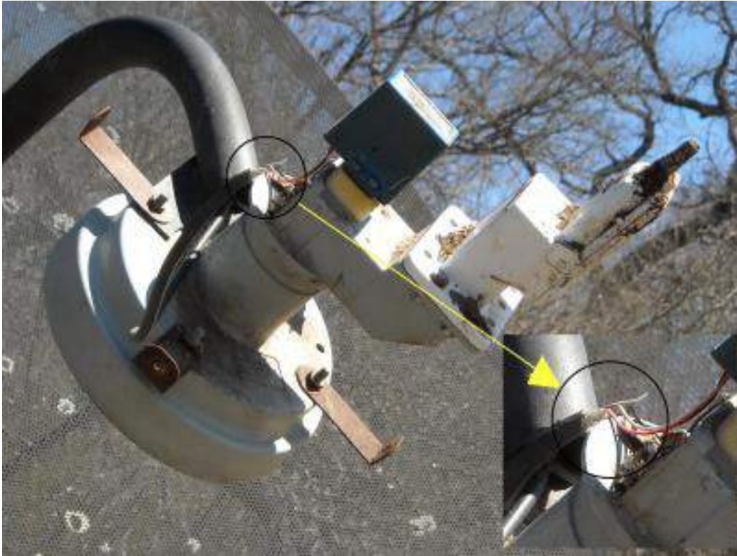
The coax had come loose from the connector
