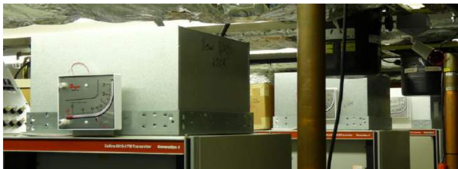
Several 831G transmitters – and more lined up in back of them!
