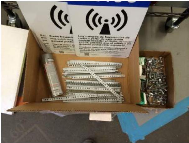
Signs, precut and pre-drilled zinc pilaster strips, and some of the zinc hardware, ready for installation
