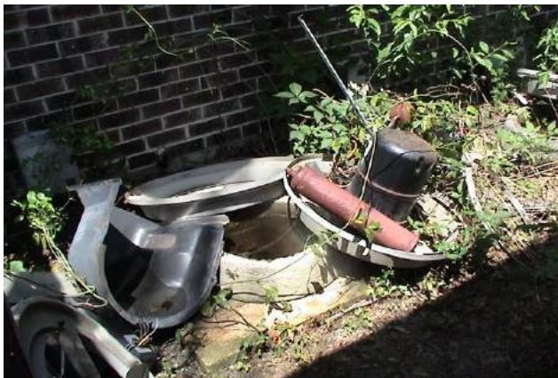
Trouble spot: HVAC units mounted "out of the way" in a narrow cubby hole between adjacent buildings.
