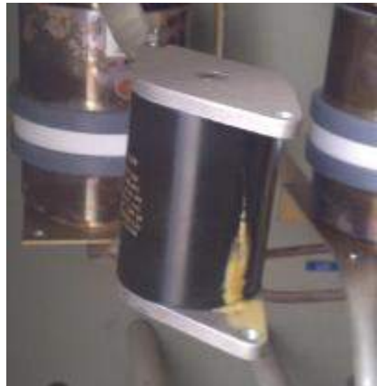
This is an ex-capacitor
