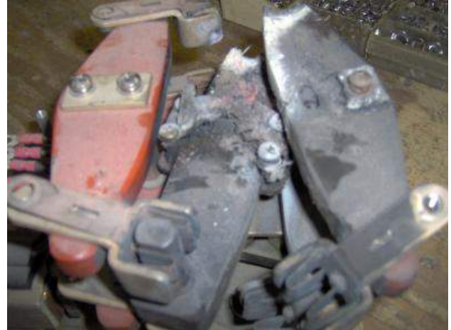
Moisture caused this contactor to burn
