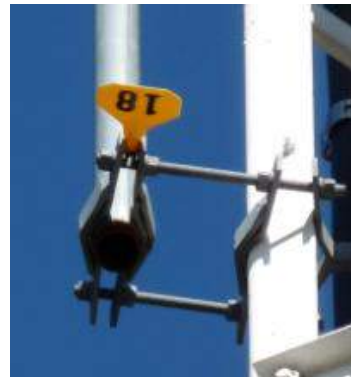
In the two pictures above, it is easy to tell which antenna is the destination for line number 18
