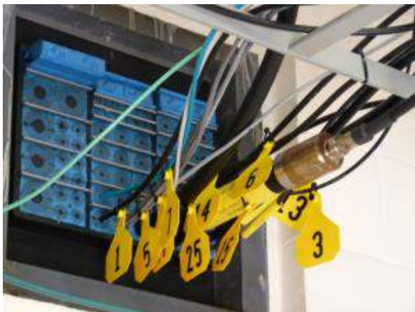
The transmitter room egress is a good point to place line numbering
