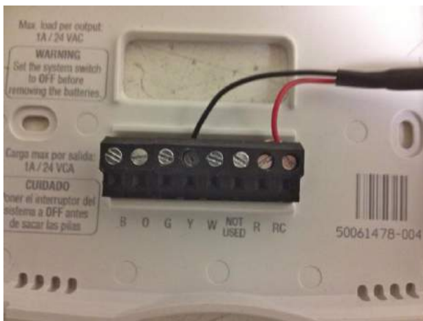
The NO wires connect to the remote control status
