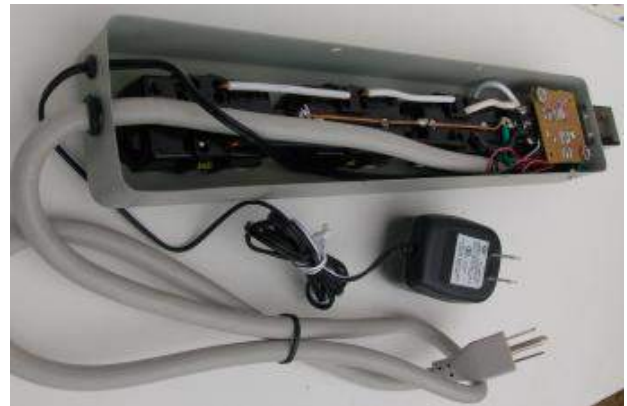
A small circuit allows remote power resetting
