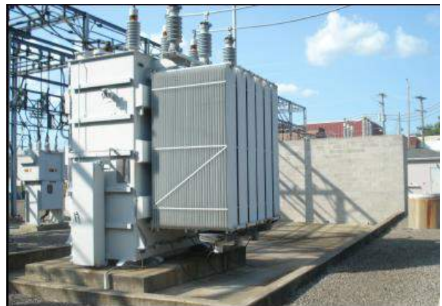
Courtesy of Grove City, PA Borough Electric
