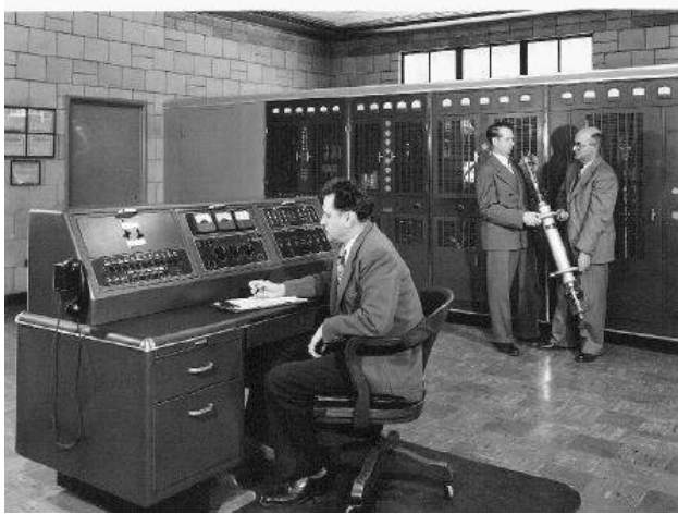
WJR's Transmitter Control with its new 50 kW Western Electric 407 transmitter.
