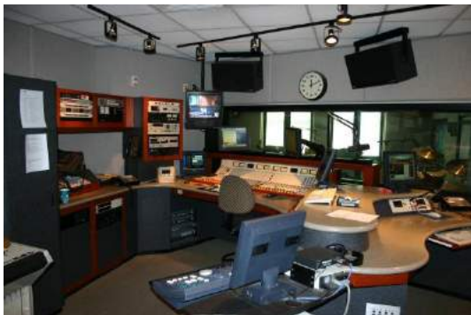
The new WJR Master Control in 2006
