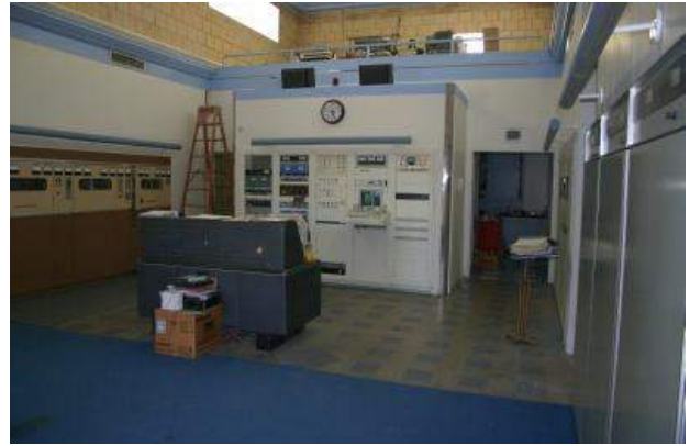
WJR's Transmitter Hall, with a DX-50 main, and 317-C2 and MW-50 backups
