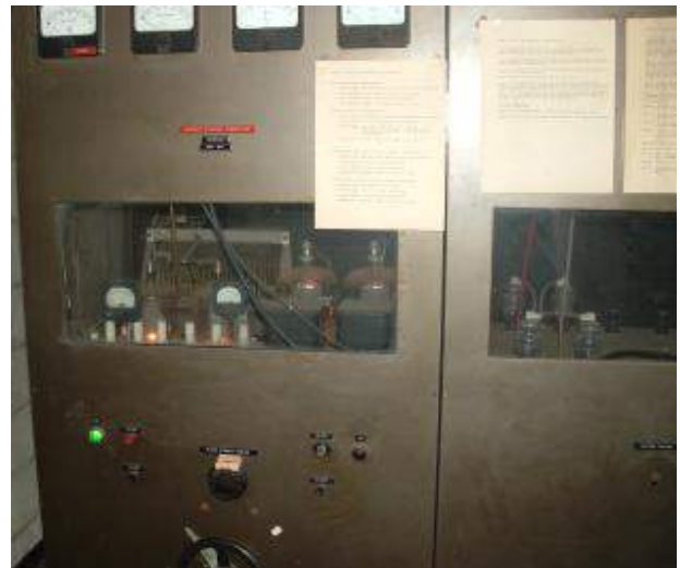
The original, homemade 1 kW WFLI transmitter
