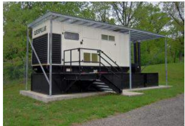
The 1 Megawatt generator, ready for action
