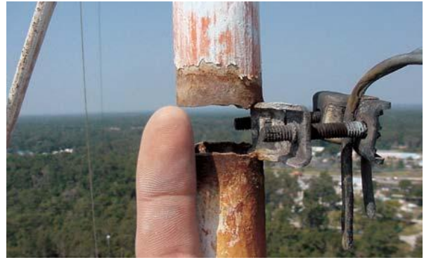
This tower leg was not designed to have a window
