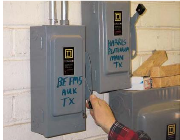
Clear marking prevents mistaking which breaker feeds which transmitter
