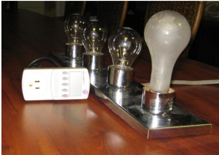
One 150-Watt and three 116-Watt lamps can be used to provide a load of up to about 500 Watts
