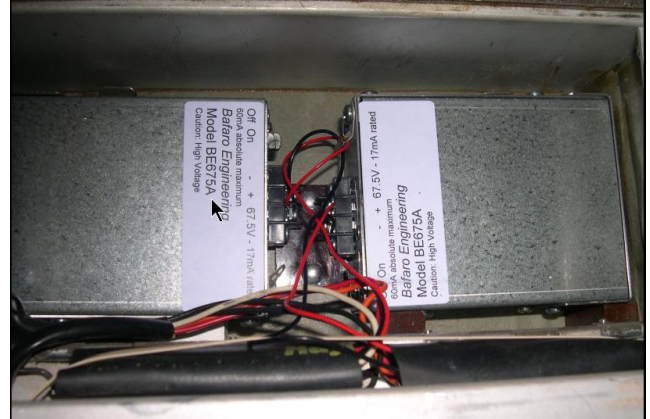
Two BE675A modules installed in an N-C 120B to replace the two B batteries.
