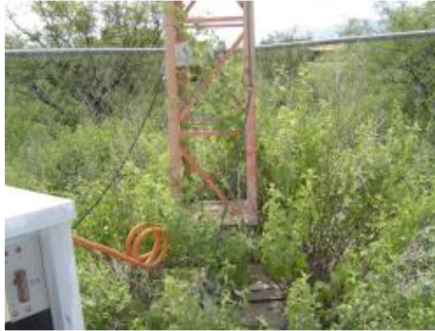
Eventually, when there is enough growth, it can even shunt power to ground
