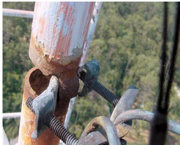
Only a tiny, buckled bit of the tower remained
