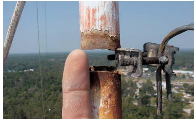
This tower leg wasn't designed to have a window
