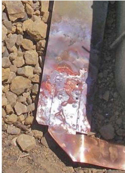
Brazed joint after copper pop rivets were installed. Yes, we ran out of 4-inch strap.
