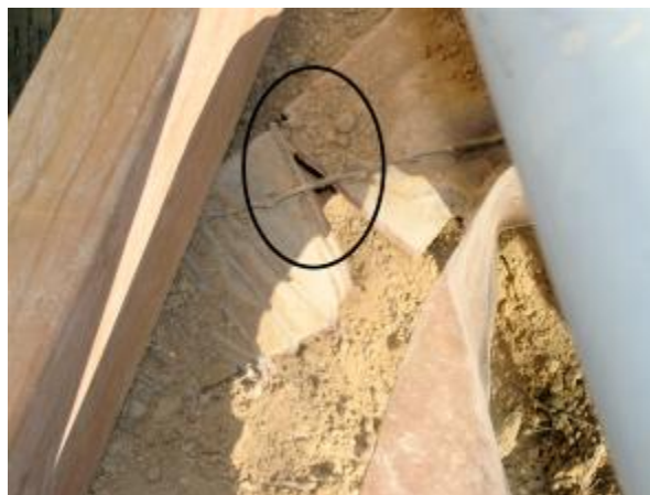
This ground strap is almost completely torn apart
