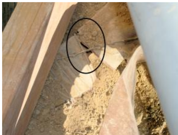
This ground strap is almost completely torn apart
