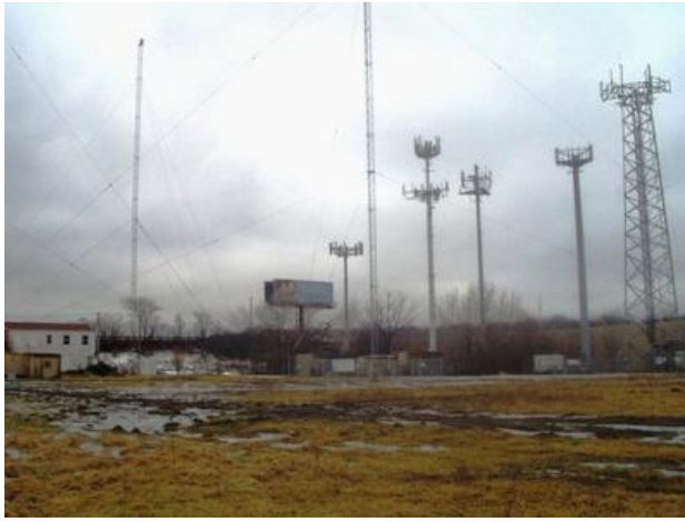
This AM directional site has several detuned cell towers in close proximity
